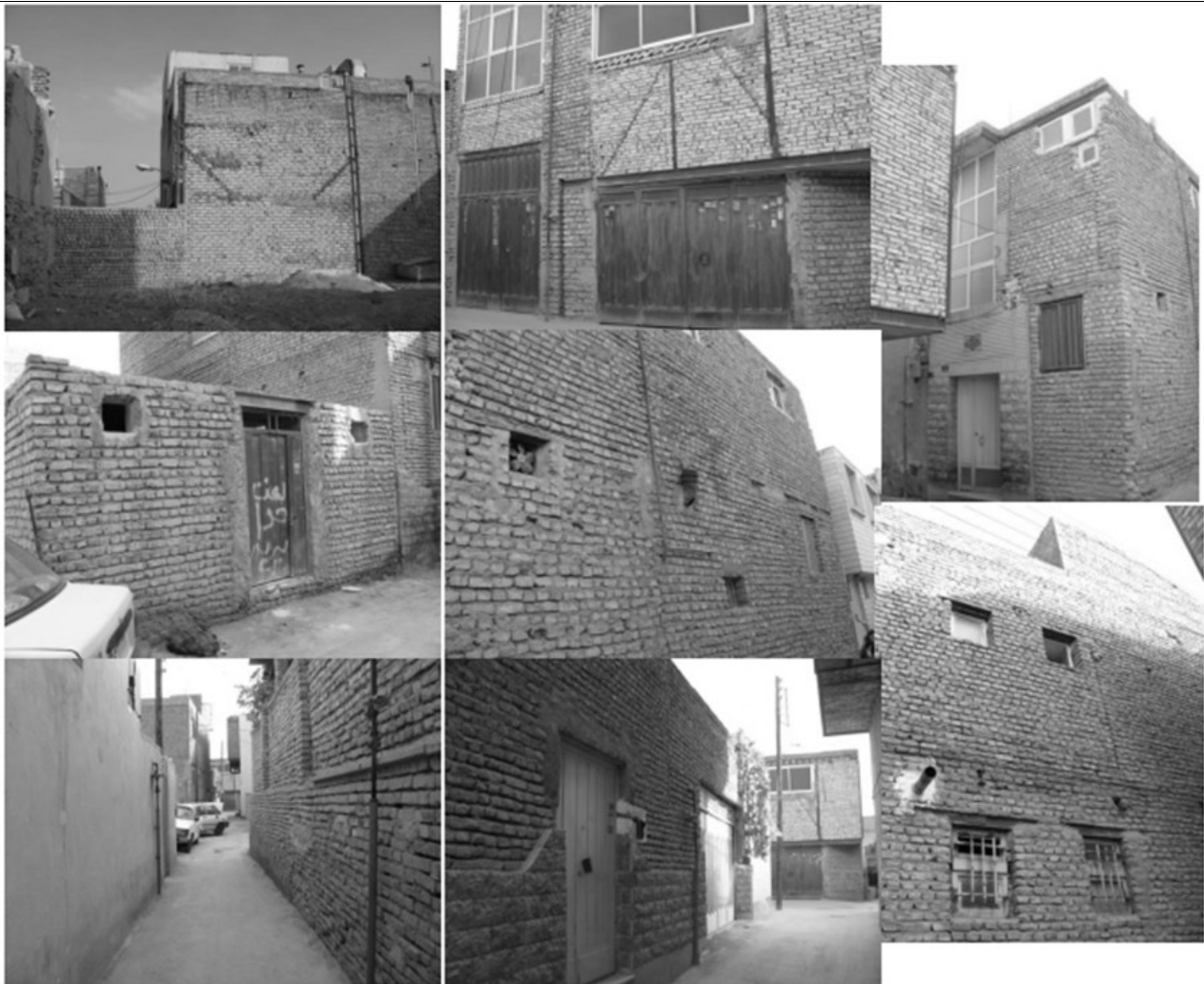
Problem 9: Buildings without façades. Solution: Design and implement a façade.
