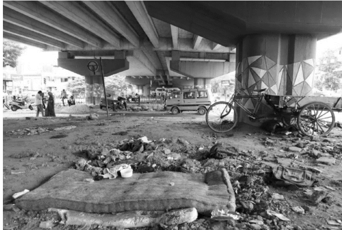
Fig 2. Sad state of Bhadrappa Layout Flyover on ORR
